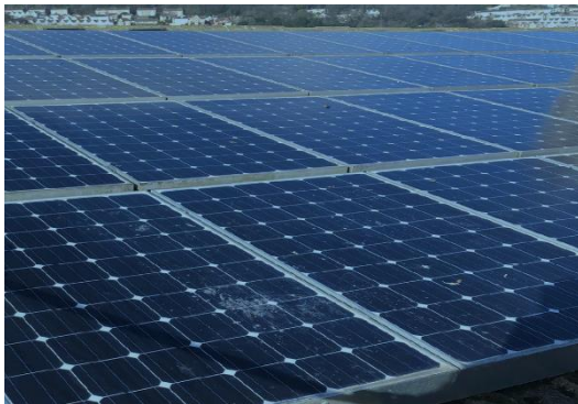
Solar PV modules installed on the Guildhall
